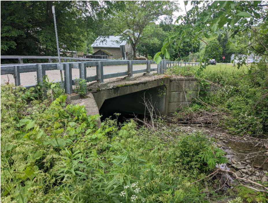
Figure 3 - Existing Structure/Box Culvert on Bentley Hill Road, 150' east of County Touring Route 66
